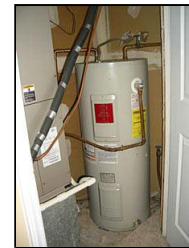
Water Heater in 02
